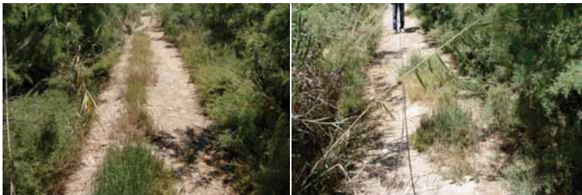
Photo 14: At 135m from western most point showing subsidence between 120 -230 m with increased vegetation in subsided area
