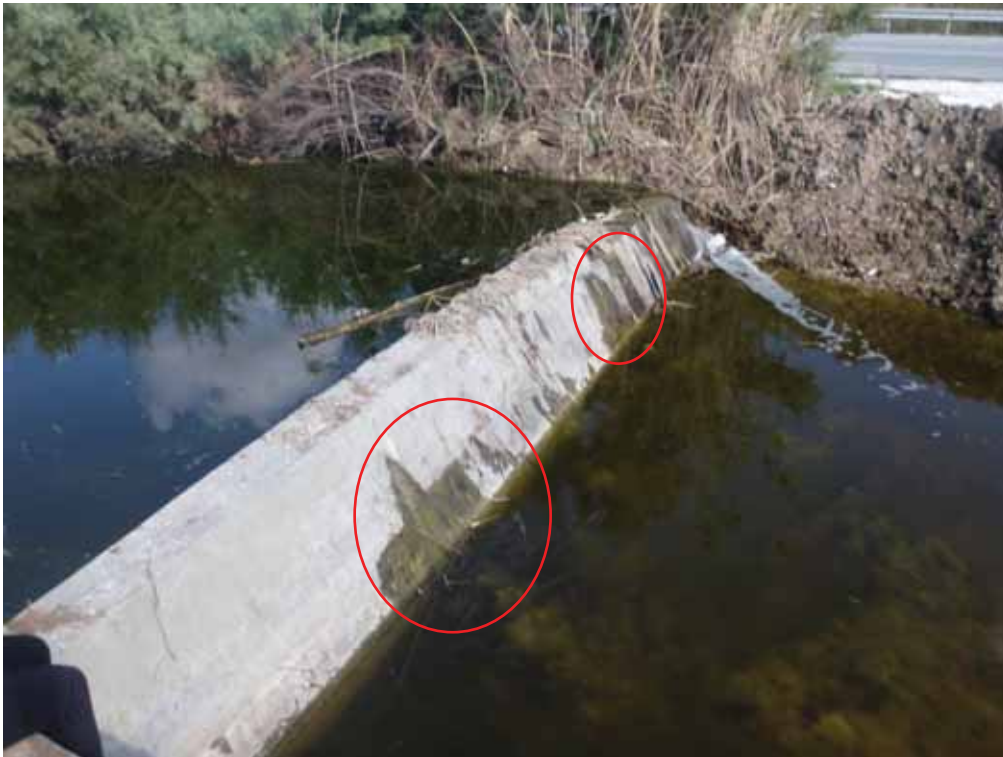
Photo 16: Minor seepage shown on the spillway wall during the spill of the lake on November 14 th 2012
