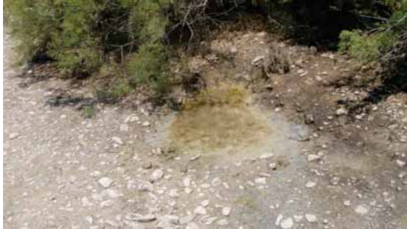
Photo 12: Non active (12/6/2012) seepage point at the lower berm of the bank at 170m from western most point
